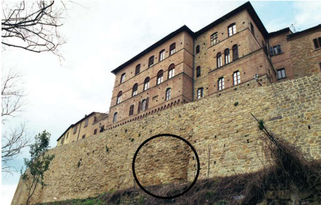
Fig. 4 - Presence of moisture before the collapse of January 2014 of the Urban walls of Volterra.
